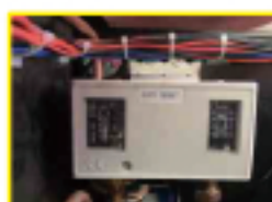
High and low voltage controllers
