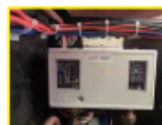
High and low voltage controllers
