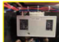
High and low voltage controllers
