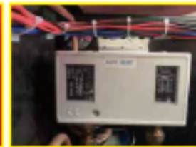
High and low voltage controllers
